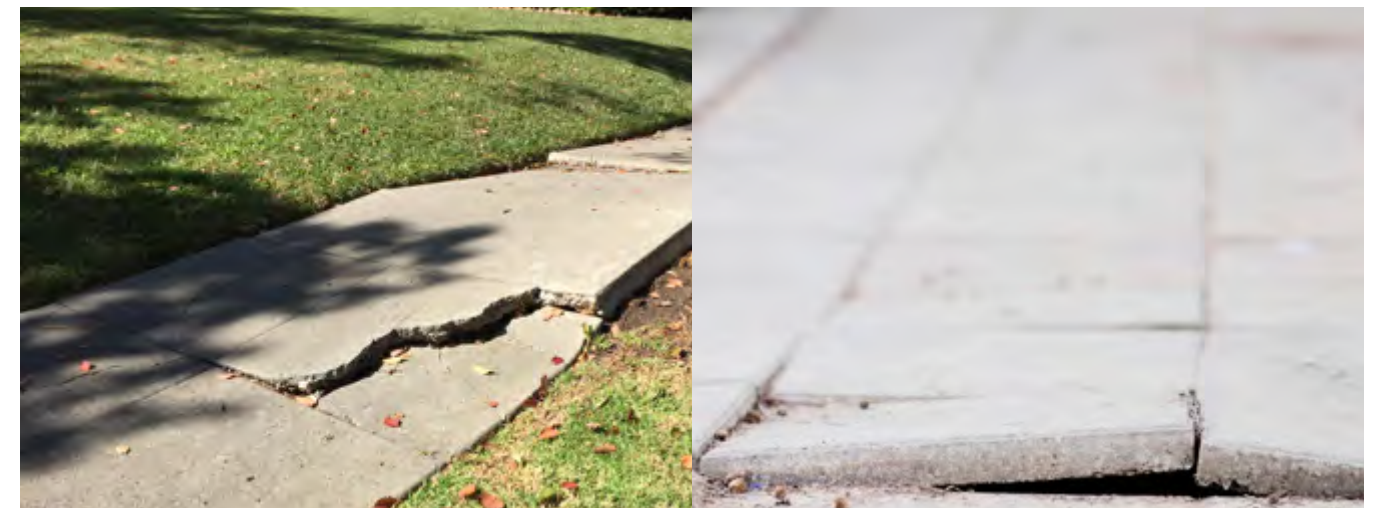
Sidewalks in need of repair
